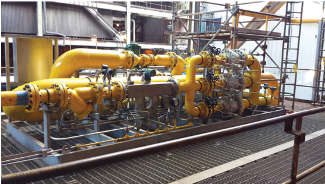
Pressure Reducing Station (rear view showing Wye strainer, Coriolis Mass Flow Meter, Pressure Regulators sized for Pin 400 psig/Pout 3-35 psig – Max flow 1,680,000 scfh).
