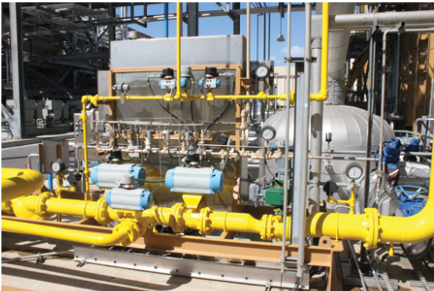
A typical duct burner fuel skid assembly
