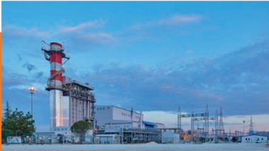
Heat Recovery Steam Generators
