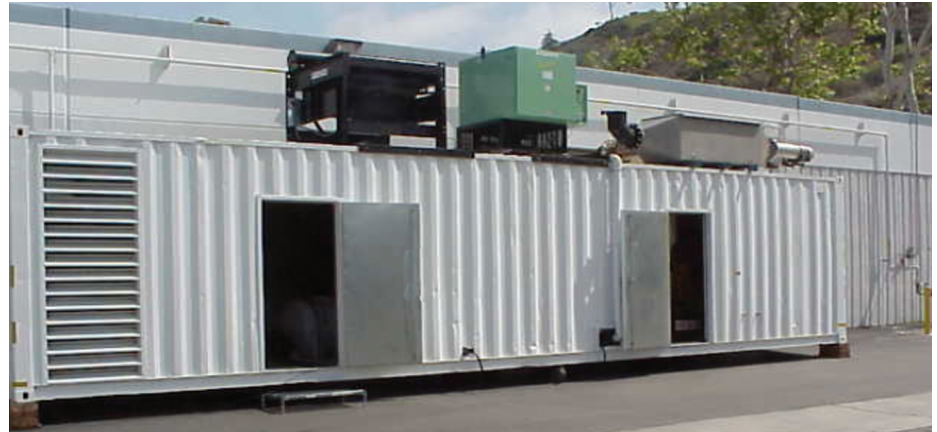
The lower rectangular housing on the extreme right (top of trailer) is the ARIS SCR system catalyst
